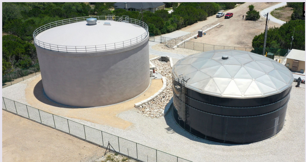
Comal County, TX — 750,000-gallon water storage tank completed at a cost of $2.2 million. One of 13 water storage projects completed, under construction, or in design.
