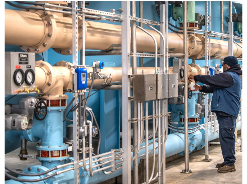
$14 million groundwater treatment facility completed in East Windsor, Connecticut
