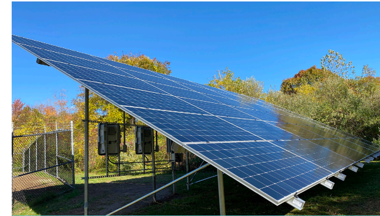
Colchester, CT – Connecticut Water completed the installation of solar panels at one of its smaller water systems which were sufficiently sized to fully meet energy requirements to pump, treat, and move water through the water system, effectively removing it from the power grid.
