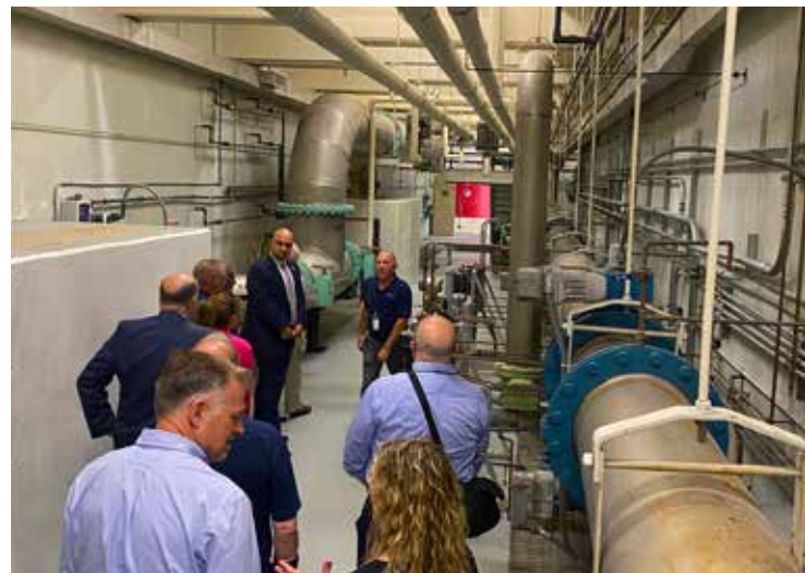
Tour of the W.C. Stewart water treatment facility for public officials in Naugatuck, Connecticut
