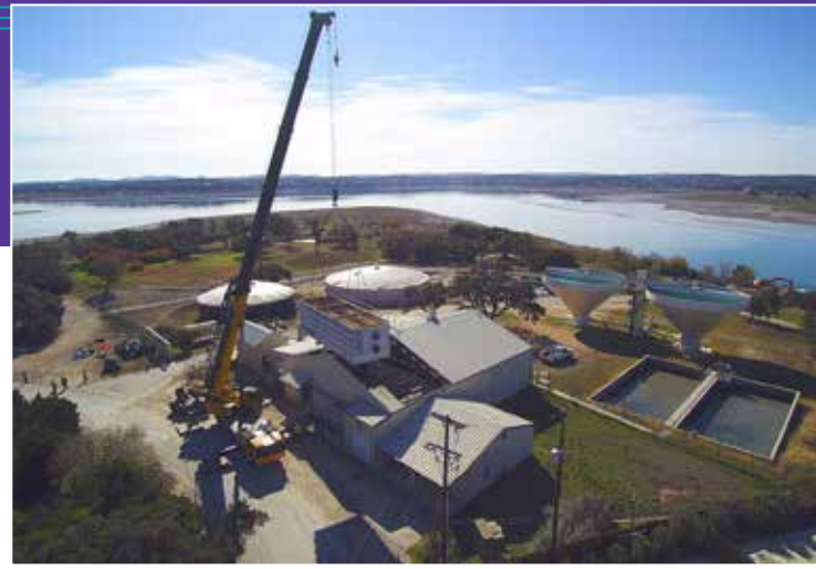
Investing in a filter replacement in Comal County, Texas
