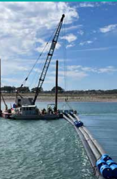
Investment in new deeper intake piping to improve resiliency for the Park Shores Water Treatment Facility in Comal County, Texas
