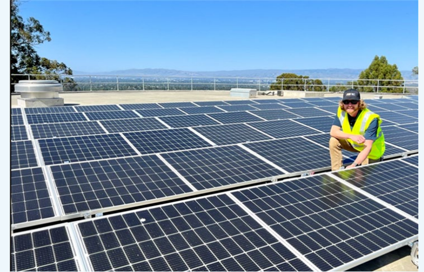
Solar generation at San Jose Water Company
