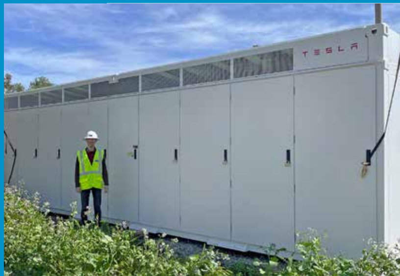
BESS on-site at San Jose Water Company's Williams Station
