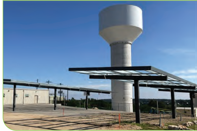
Construction of parking canopies at Texas Water with solar generation integrated into the roofs; similar solar canopies are online at San Jose Water.
