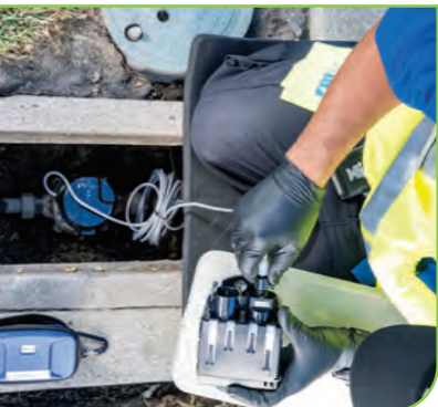
More than 20,000 smart meters have been installed at San Jose Water, with the rest expected to be installed by 2027.
