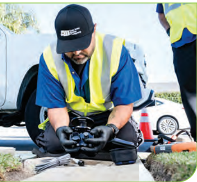
Installation of advanced metering infrastructure (AMI) at San Jose Water that enables smart meters to provide near-real-time usage information.
