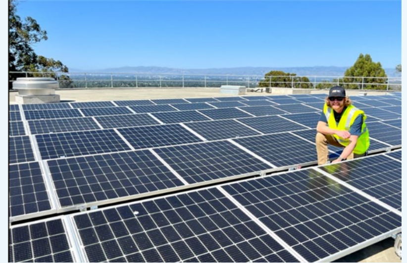
Solar generation at San Jose Water Company
